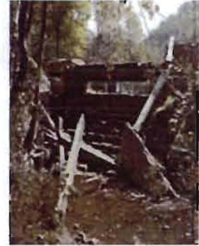
Civilian Conservation Corps-era damaged dam
